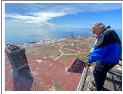
Chuck Scheckel examines roof damage on the Pilot Island lighthouse. Photo by Tim Sweet.
