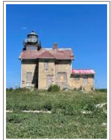
The Pilot Island lighthouse roof after repairs, August 15, 2023. Photo by Bill Peterson.
