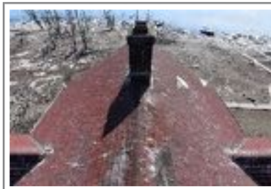
The Pilot Island lighthouse roof shingle damage, May 2023. Photo by Chuck Scheckel.
