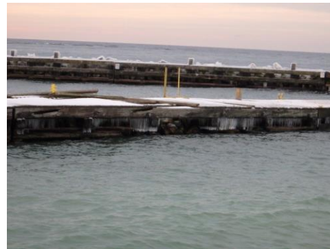
Figure 2: Examples of the dock damage.
