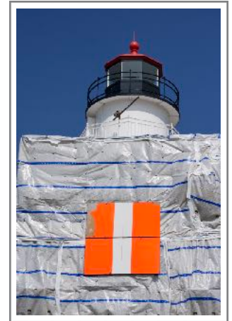
Rear range light with temporary dayboard shrouded to contain hazardous waste.
