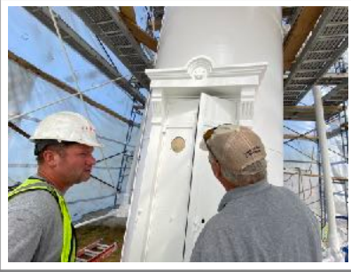
Billy Winkleback of Mihm and Chuck Sheckel, FOPPI Historic Preservation team leader, inspect the paint job on the rear range light.
