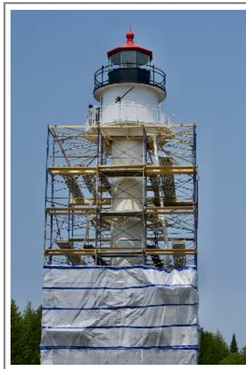
Scaffolding surrounds the range light, which is shrouded to contain paint and dust.
