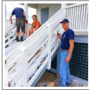
Paul, Ginnie, and Dallas paint the porch railing on the crew quarters.
